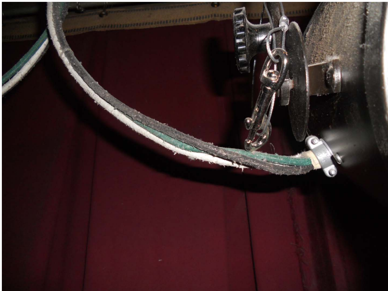
Example of asbestos wire insulation.
