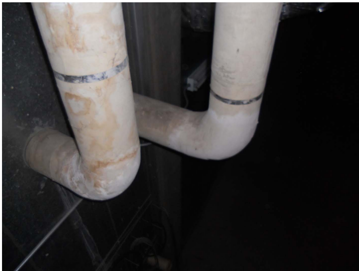
Example of thermal system insulation mudded joint fittings.
